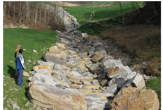
“Reclamation” involves turning a vibrant stream into a sterile rock-lined drainage ditch such as this one at the head of Island Creek in Pike County.
